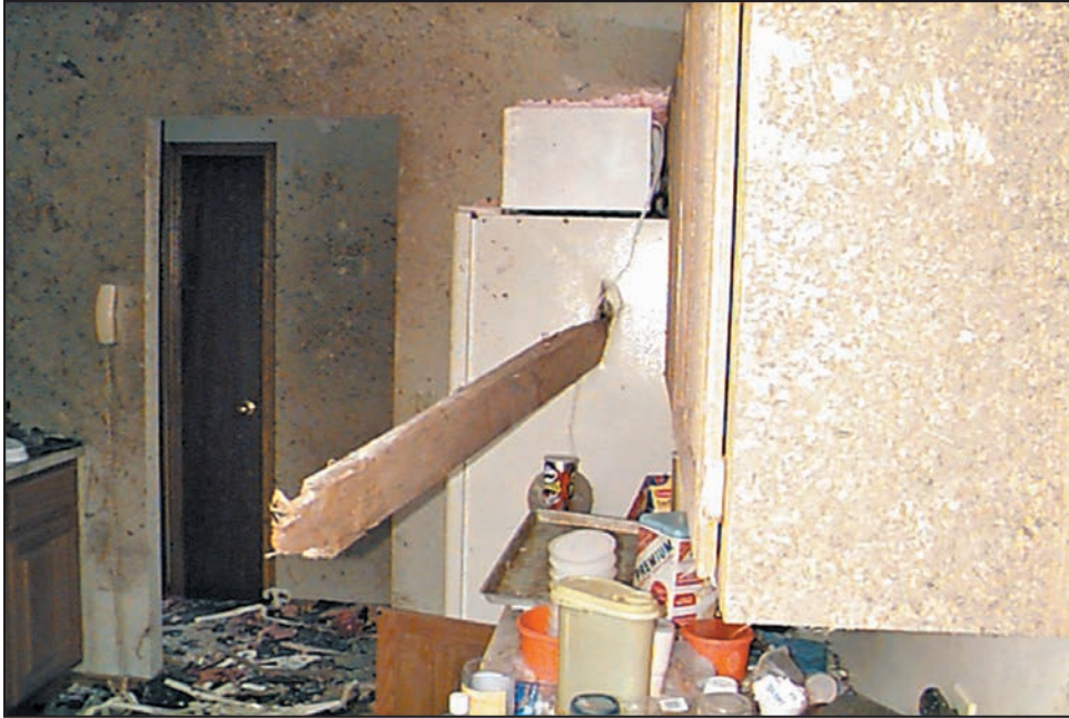
Figure B8-11. Refrigerator pierced by a 2x6. The portion of the 2x6 that is visible was 4 feet 8 inches long. It went several inches into the freezer compartment.
