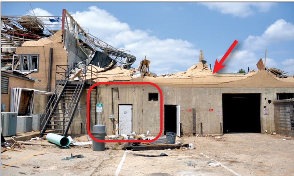
Figure B3-14. Collapse hazard: the story above an Emergency Operations Center collapsed. Masonry walls (red arrow) and part of the roof structure fell onto the second story floor slab above the EOC (Tuscaloosa, AL, 2011 tornado) (SOURCE: FEMA P-908, RECOVERY ADVISORY 6)
