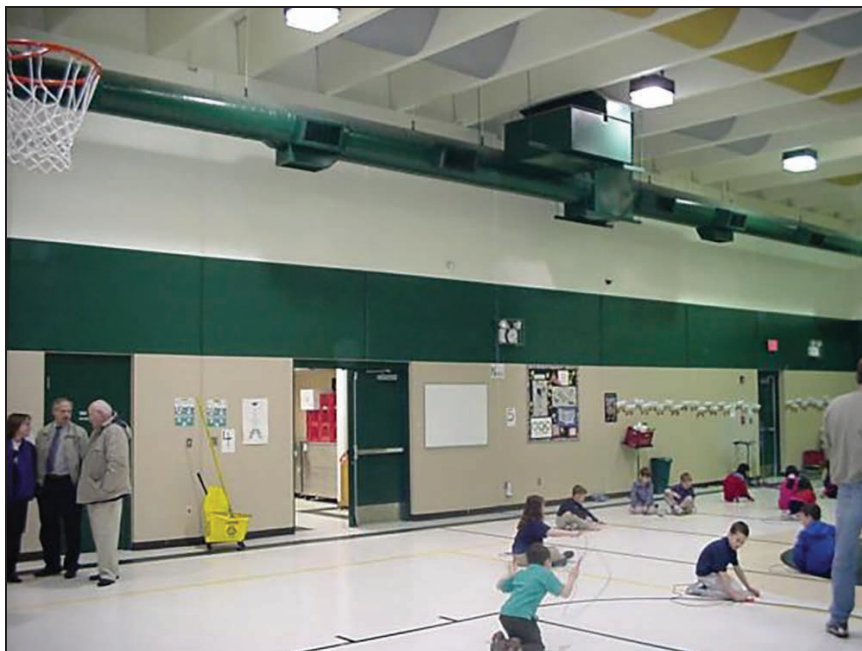
Figure A4-1. Example of a multi-purpose safe room also used as a gymnasium
