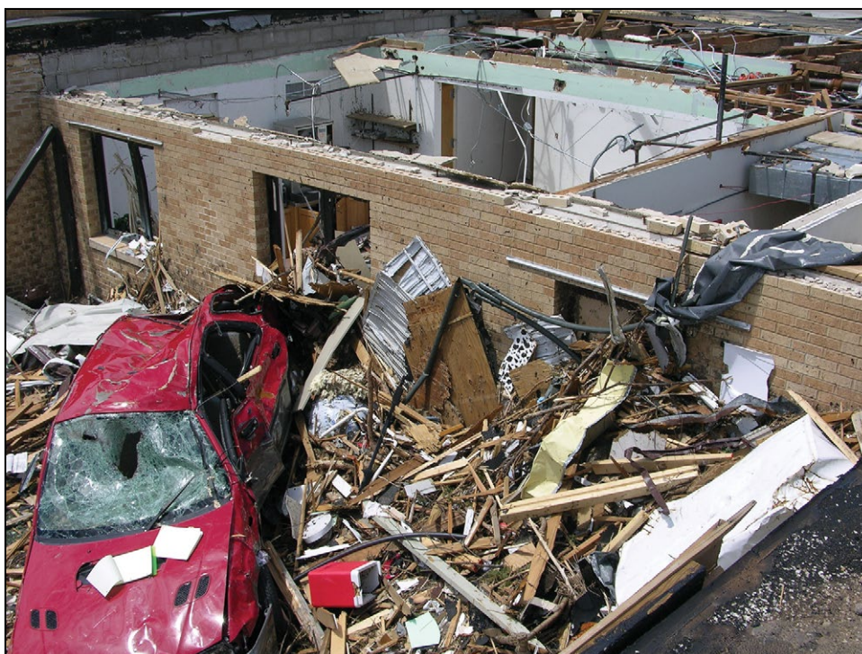
Figure B8-10. Representative quantity, size, and type of debris that is often generated by a strong or violent tornado. The building damage at this site was indicative of an EF3 tornado. (Greensburg, KS, 2007) (SOURCE: FEMA P-577)
